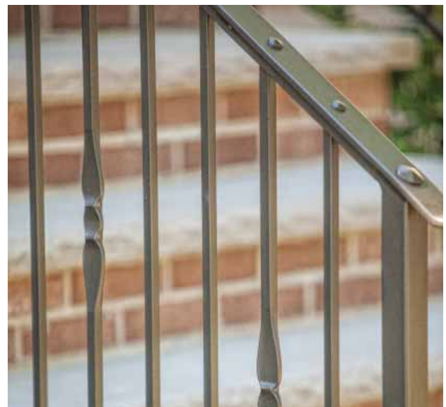
Roanoke (Railing has rivets through handrail)
