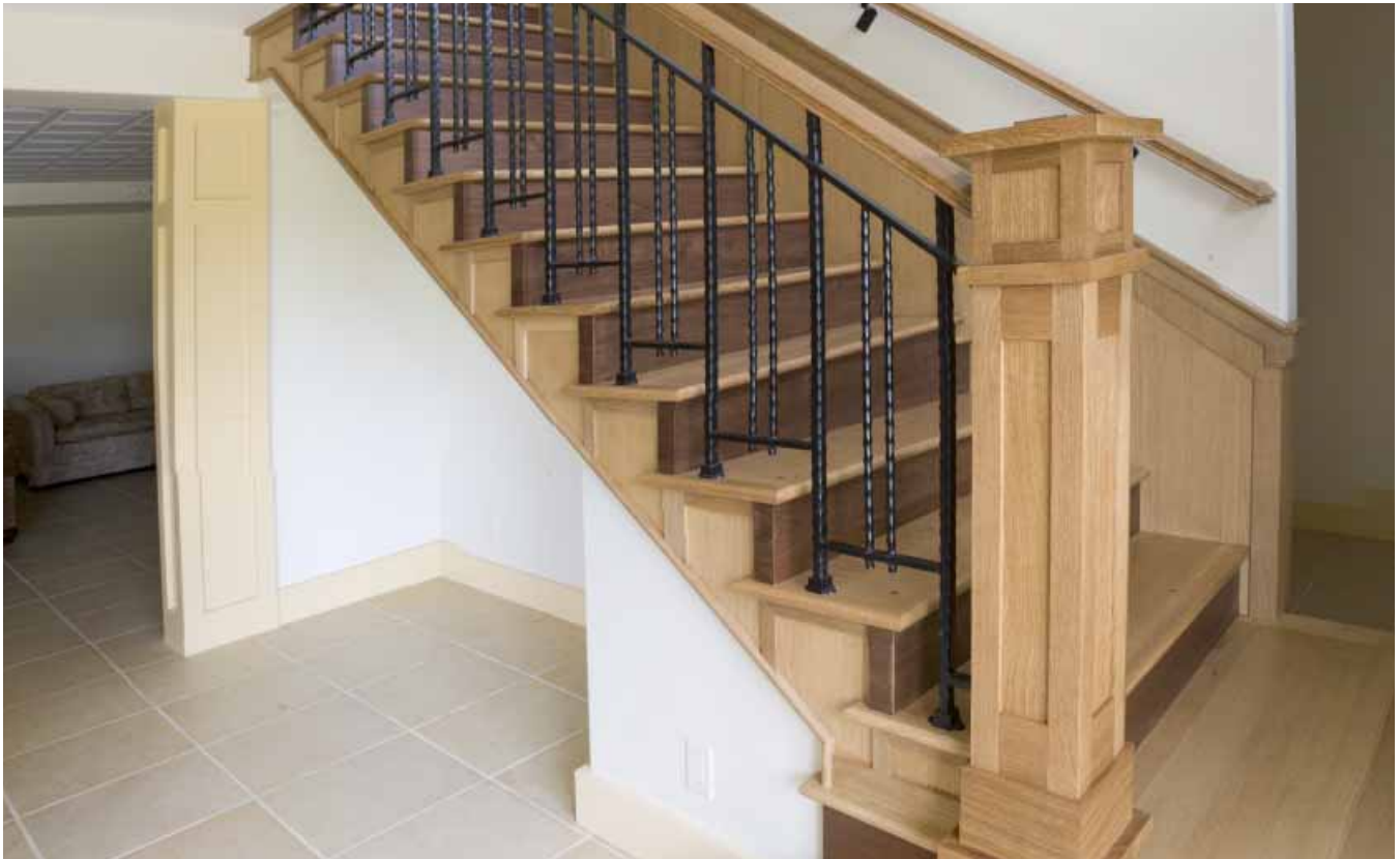
Arts & Crafts Style railing in Maryland
